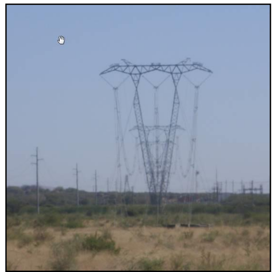
Plate 2: A 520B Guyed Vee tower
