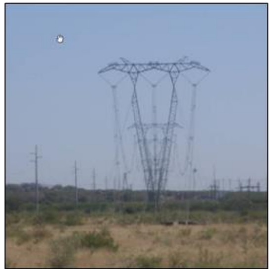
Plate 2: A 520B Guyed Vee tower
